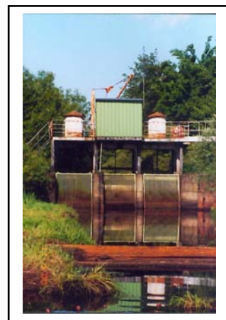
Station de pompage
